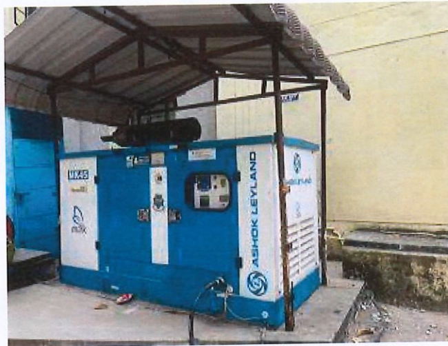
Figure 5-3: Diesel Generator (DG) sets
