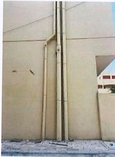
Figure 8-7: Pipelines for rain water
