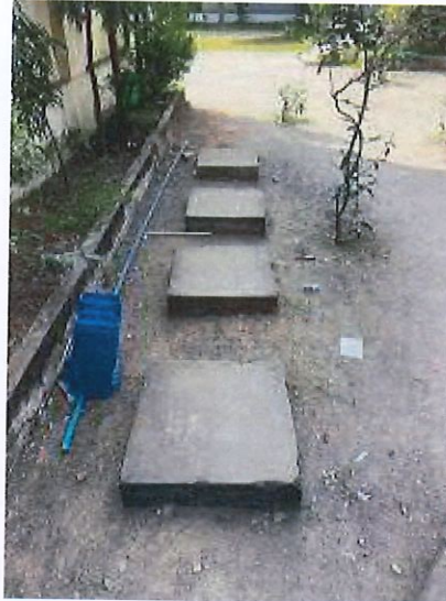
Figure 5-10: Earth pits with closures
