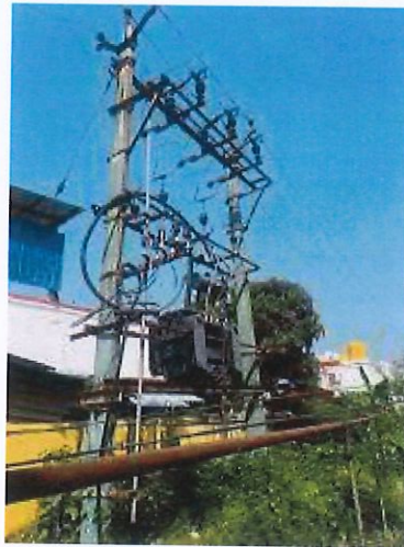
Figure 5-1: Transformer unit near campus
