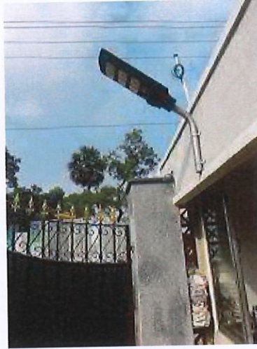
Figure 5-9: Solar LED Street lights
