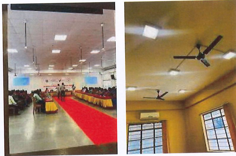
Figure 5-7: Use of LED fixtures
