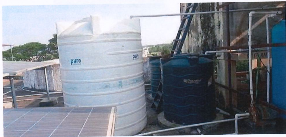
Figure 4-8: RO Reject storage tank
