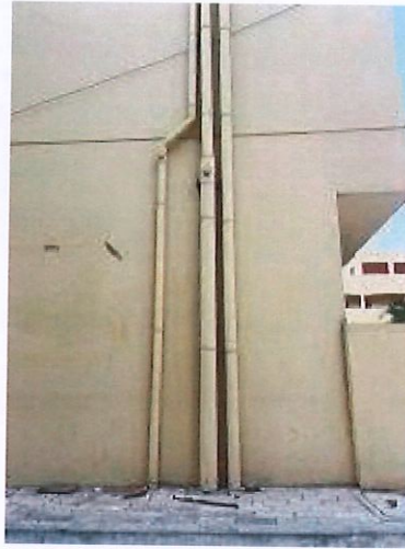
Figure 4-9: Pipelines for rain water
