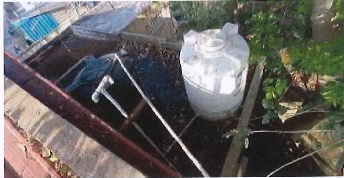
Figure 4-4: PVC overhead tanks in Hostel, Boy's toilet & canteen terrace
