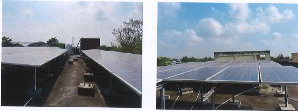
Figure 5-6: SRTPV modules at college terrace
